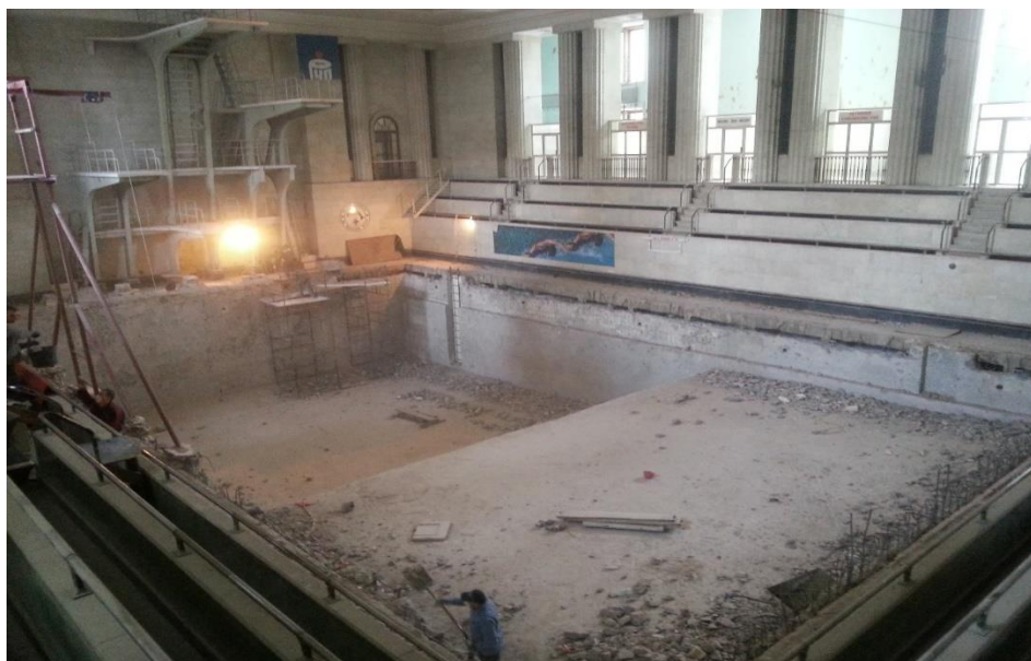
Fig. 3. The Palace of Youth in Warsaw, the indoor swimming pool in 2014, under modernisation and renovation works (source: Bartłomiej Krynicki, 2014)
